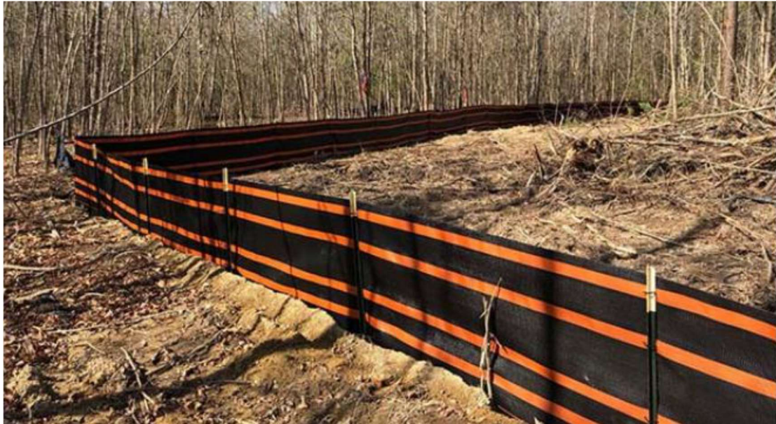
Figure 7. Example of Silt fencing.
